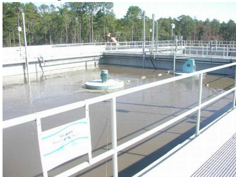
The tanks where the wastewater is stirred and injected with water is where most of the work of the plant occurs.
